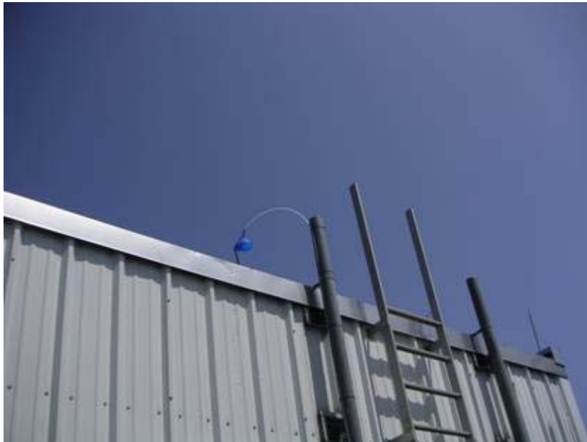
FIGURE A.8: Ozone analyzer inlet, Bank of Oklahoma Tower; inlet was protected from water intrusion by a downward-placed funnel (blue object in photograph to the left of the access ladder).
