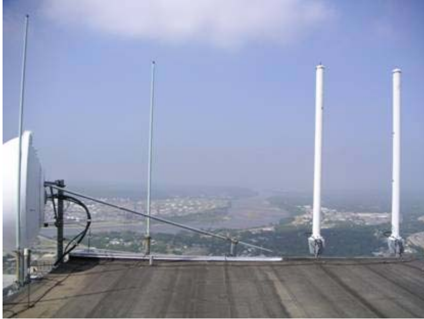
FIGURE A.7: Roof of the City of Tulsa Communications Facility, Bank of Oklahoma Tower; 210-meter ozone analyzer inlet was mounted on an adjacent pole on this structure.
