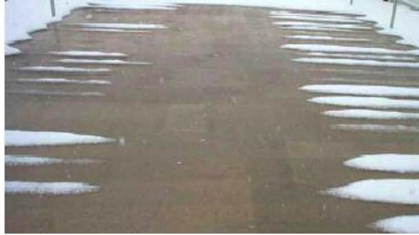
Figure 2-4 Picture showing ‘stripes’ of snow on a heated bridge surface.
