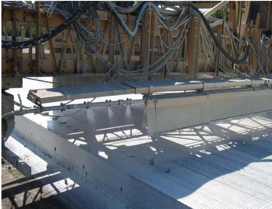
Figure 3 - 1: The power-driven spray to perform a uniform application on a tinned surface (Ye et al, TxDOT 2009)
