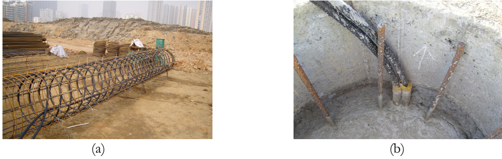
Figure 2 Circulation pipe intertwined with steel cage and concrete pouring of the pile foundation
