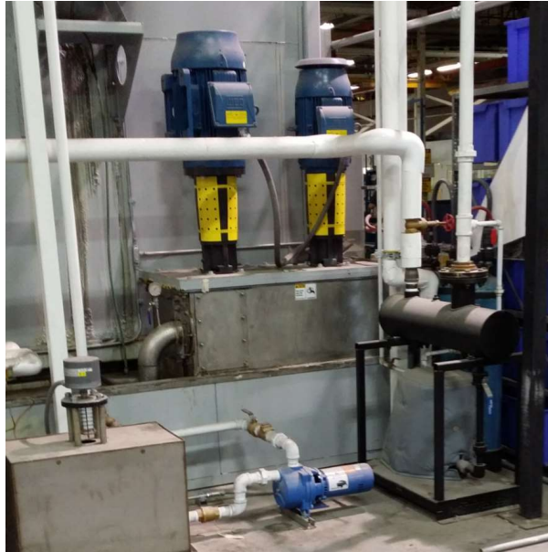
Figure 4-25: Picture of Back of Parts Washer and Drain Pump
