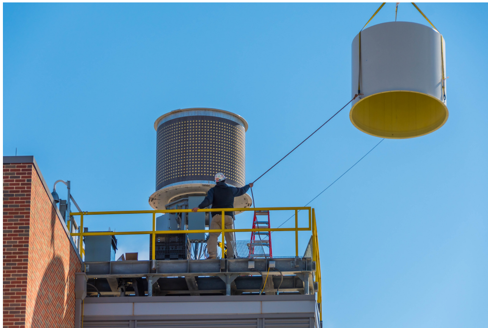
Figure 3.1: CPPAR and its radome installation on the roof of the Radar Innovations Laboratory.
