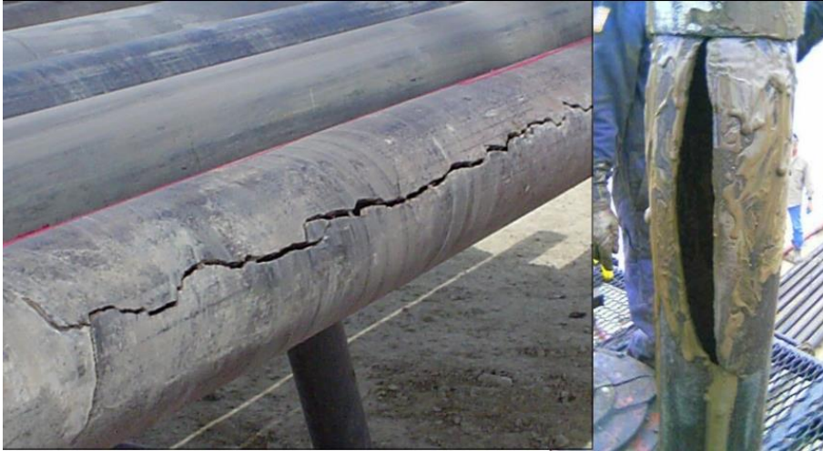
Figure 17. Example of split failures in casing (Magill, 2013)
