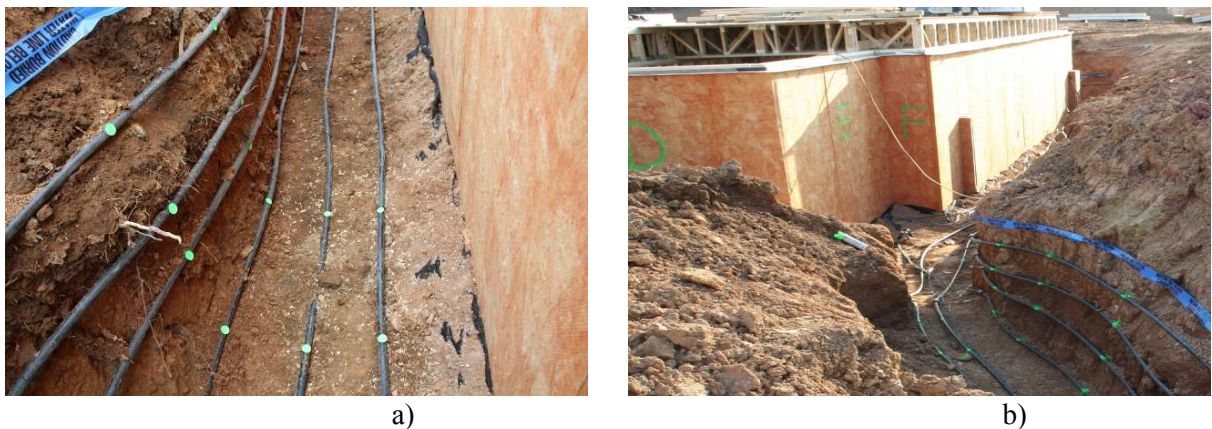
Figure 1.1: FHX. a) In basement excavation, b) extended into utility trench, (photo: Im 2009)
