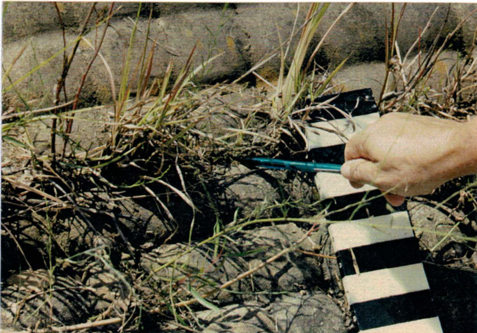
Illustration 4 Vegetative growth in longitudinal cracks
