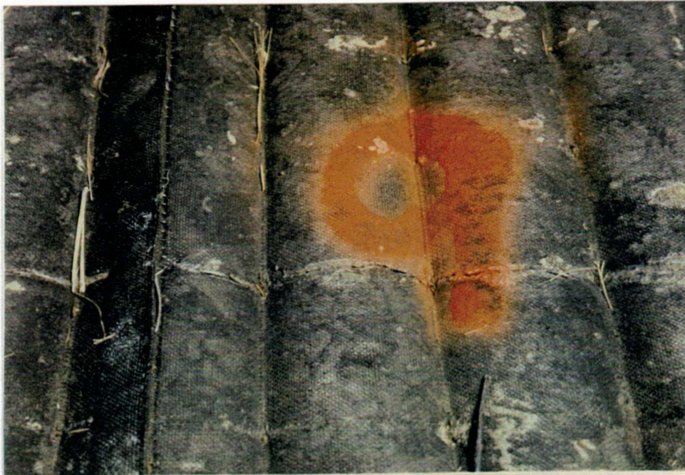
Illustration 7 Section 9 - Showing cracking at seam line
