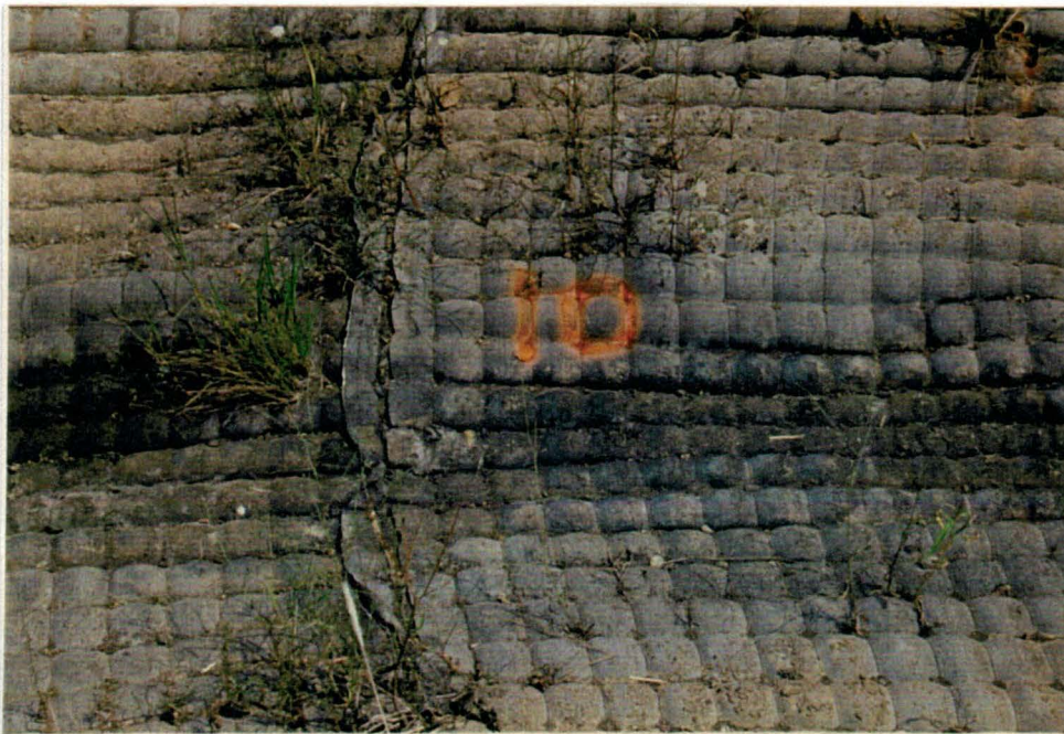
Illustration 6 Section 10 - Showing seam separation
