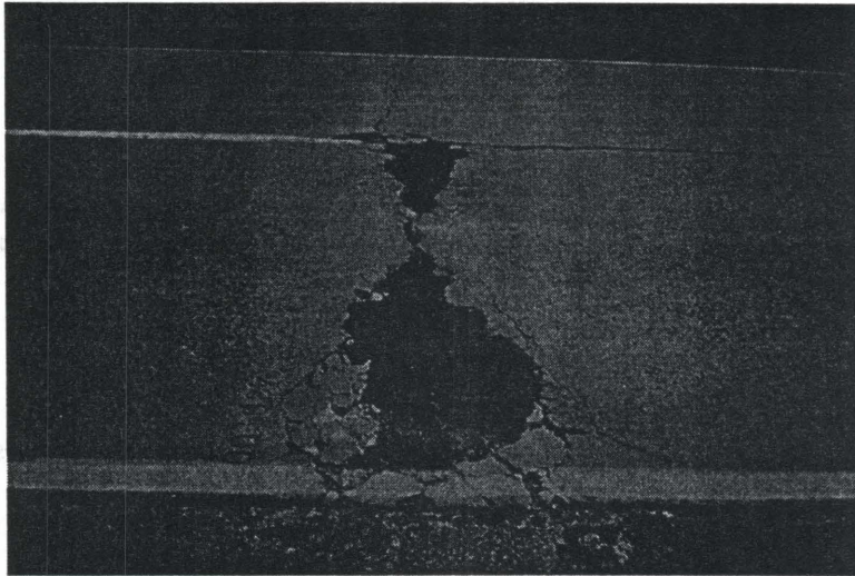
Figure 1. High-severity transverse crack.
