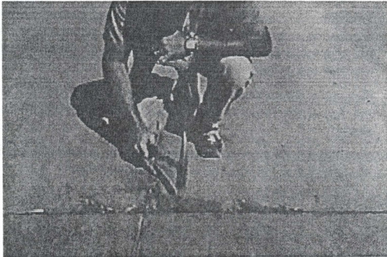
Figure 18. Sounding with ballpeen hammer.
